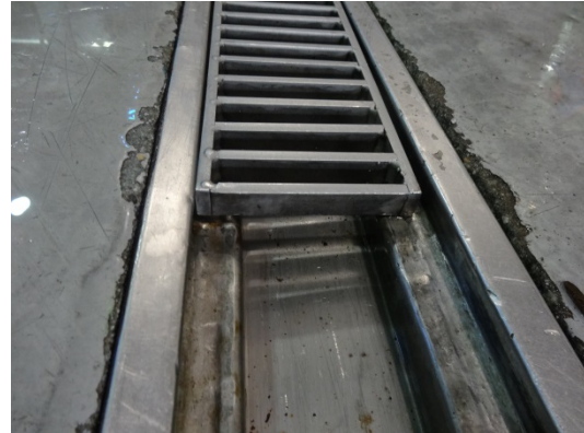
Figure 3 - Flaws in the floor-drainage connection
